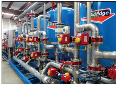
ADEGE PACKAGED UNITS (APU)
