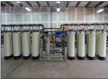
MODULAR TREATMENT SYSTEMS
