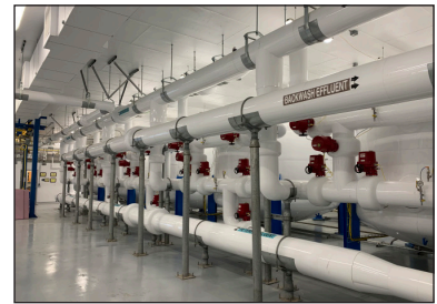
LARGE MODULAR TREATMENT SYSTEMS
