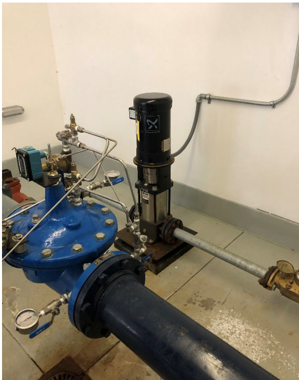
Figure 1 - CLAVAL PRV station (Hydraulically controlled), SCADA and data collection
