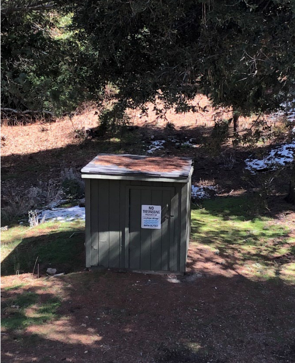
1 vertical well at HQ
