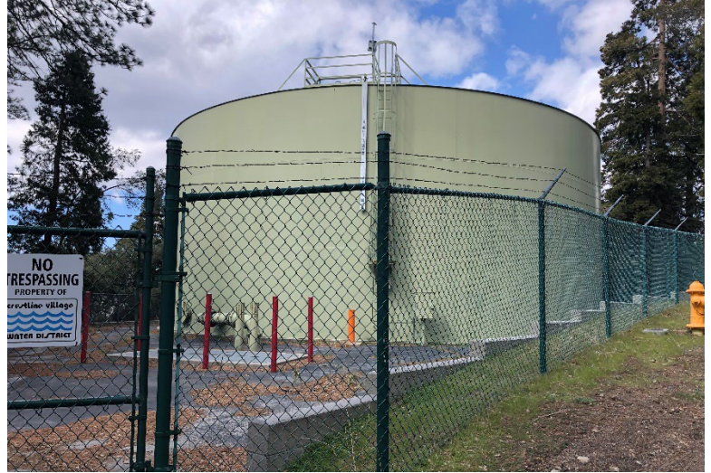
Figure 2 – Old Mill Tank - Just SCADA – some outside coating failures
