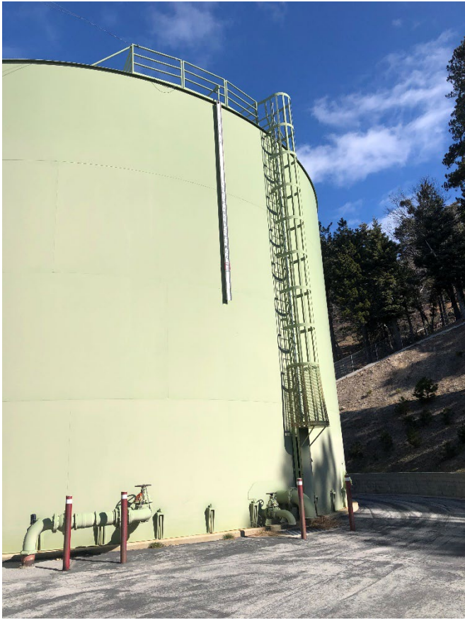
Figure 3 - 2 tanks SCADA and Data Collector
