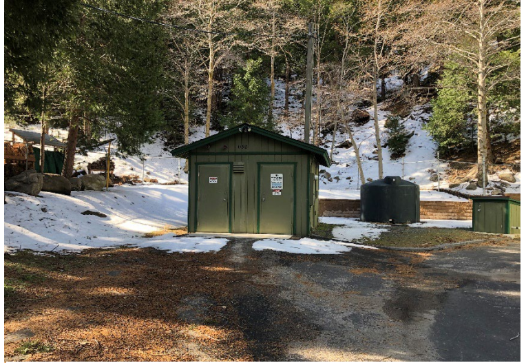
Figure 2 – vertical well and chlorine station
