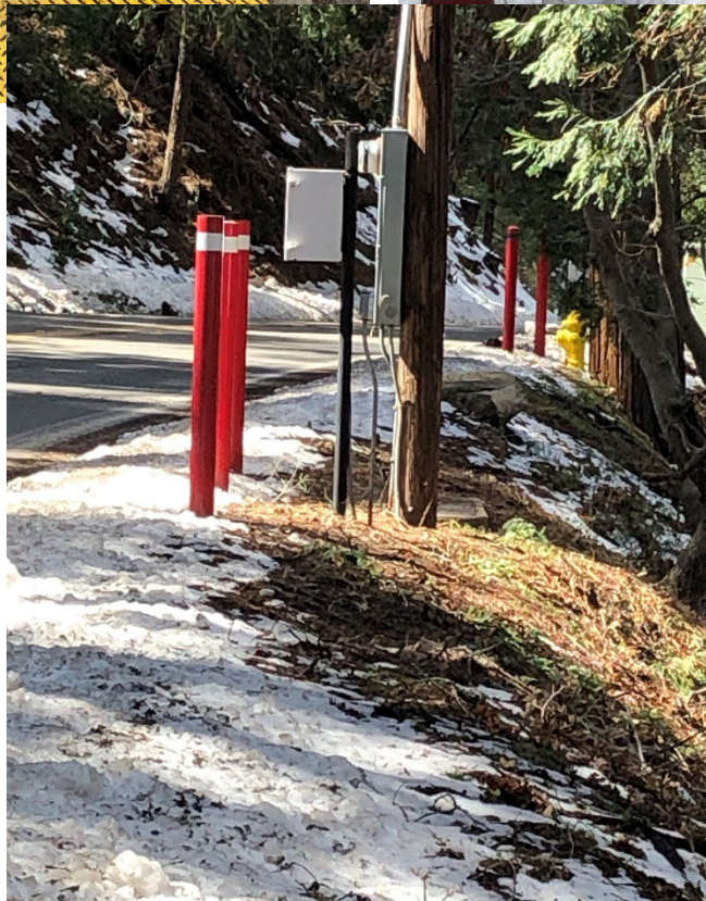
Figure 3 - CLAWA intertie, SCADA flow capability
