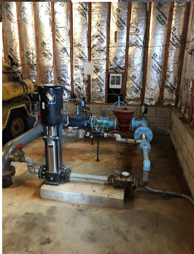
Figure 3 - CLAVAL PRV station (Hydraulically controlled) with Pump
