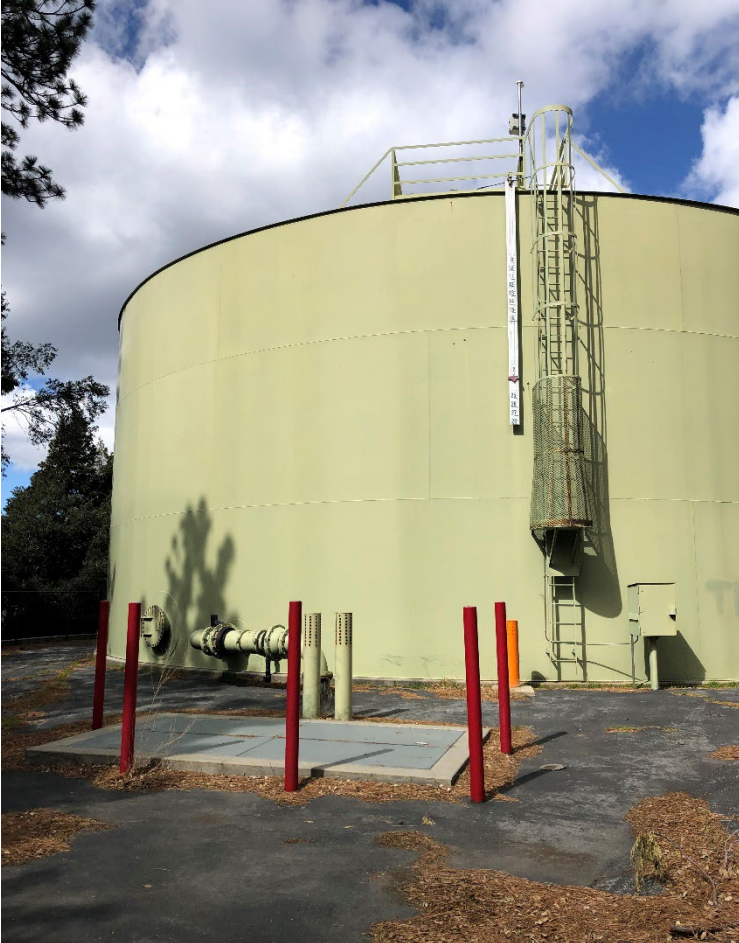
Figure 1 – Old Mill Tank - Just SCADA – some outside coating failures
