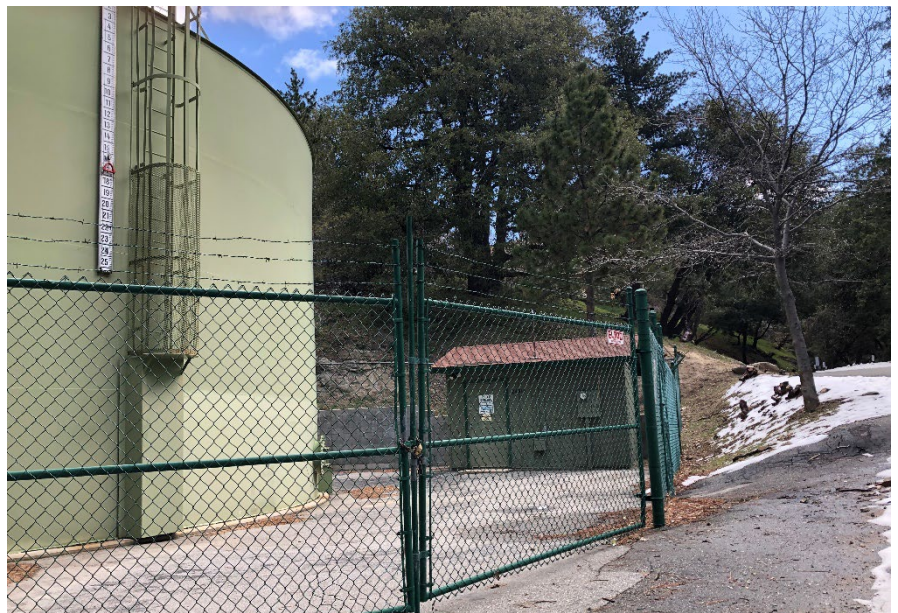
Figure 2 - CLAVAL PRV station (Hydraulically controlled), SCADA and data collection
