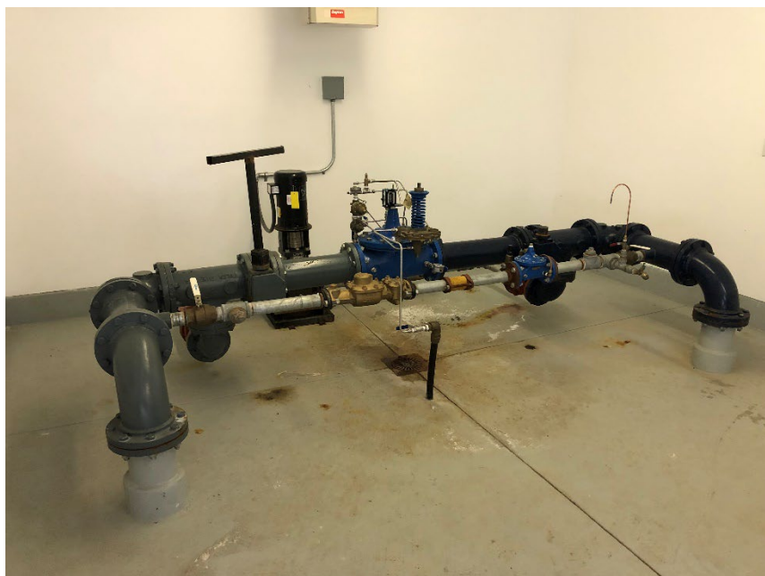
Figure 2 - CLAVAL PRV station (Hydraulically controlled), SCADA and data collection
