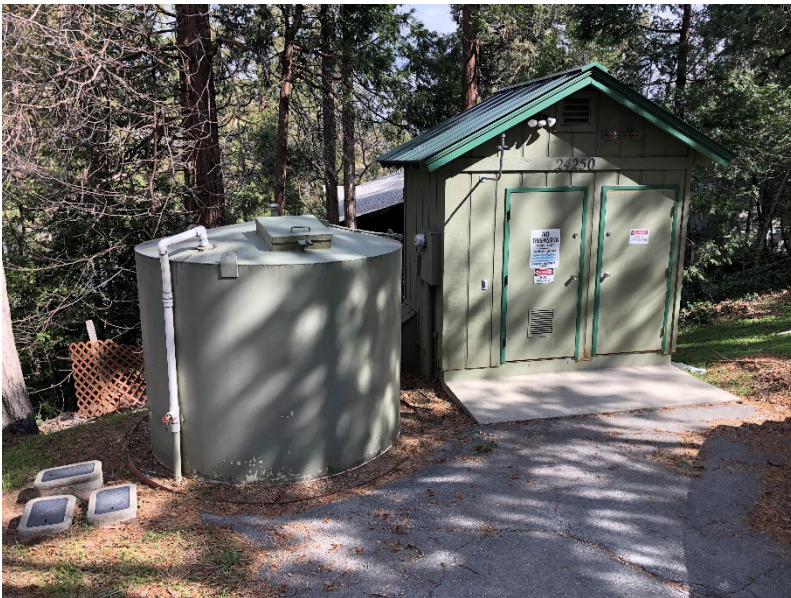
Horst – 3 horizontal Wells Chlorine and Phosphate
