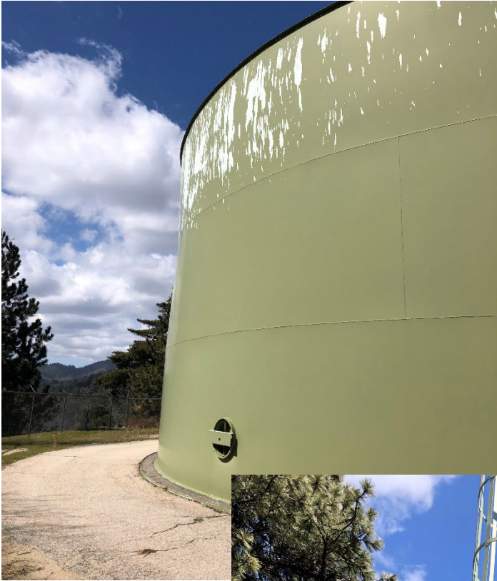
Brookside Tank Figure 3 – SCADA & Data Collection, outside coating should be evaluated
