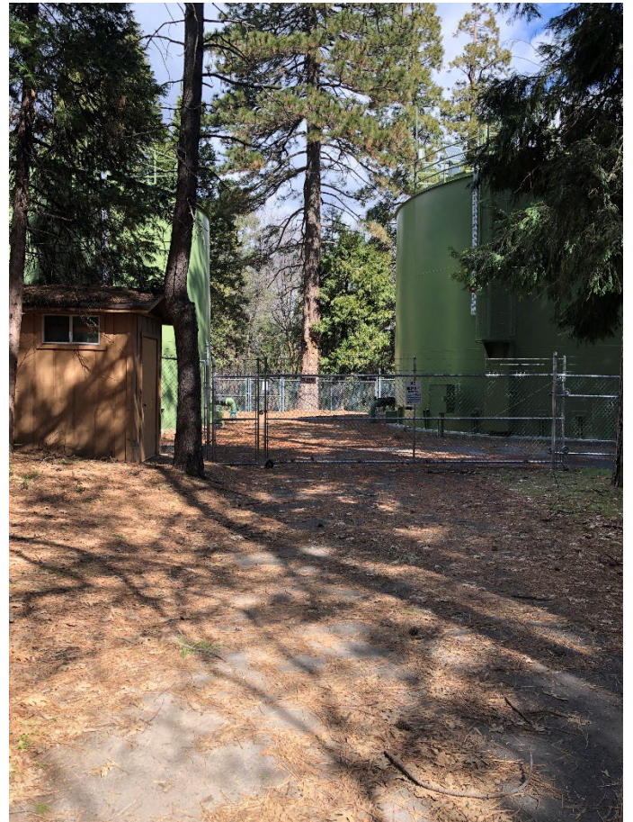
Figure 2 - two tanks, SCADA and data collector
