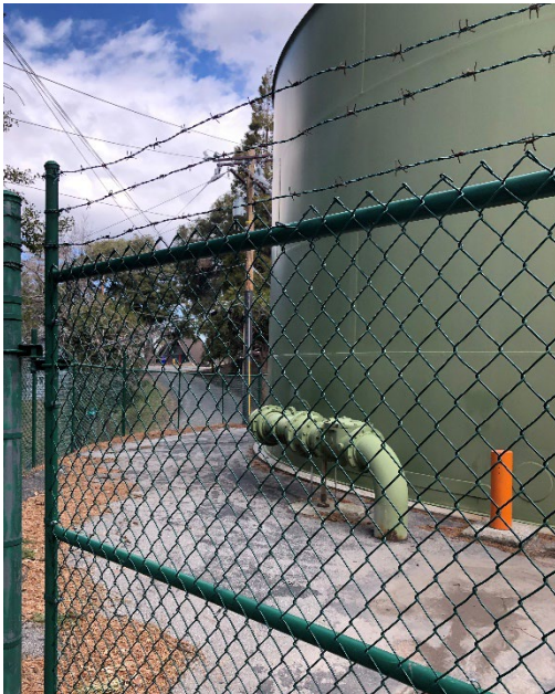
Figure 1 - CLAVAL PRV station (Hydraulically controlled), SCADA and data collection
