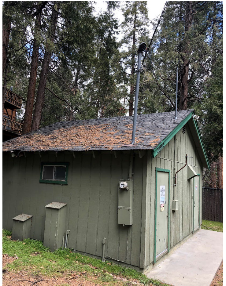
Pioneer Well – 4 horizontal wells, chlorine, phosphate
