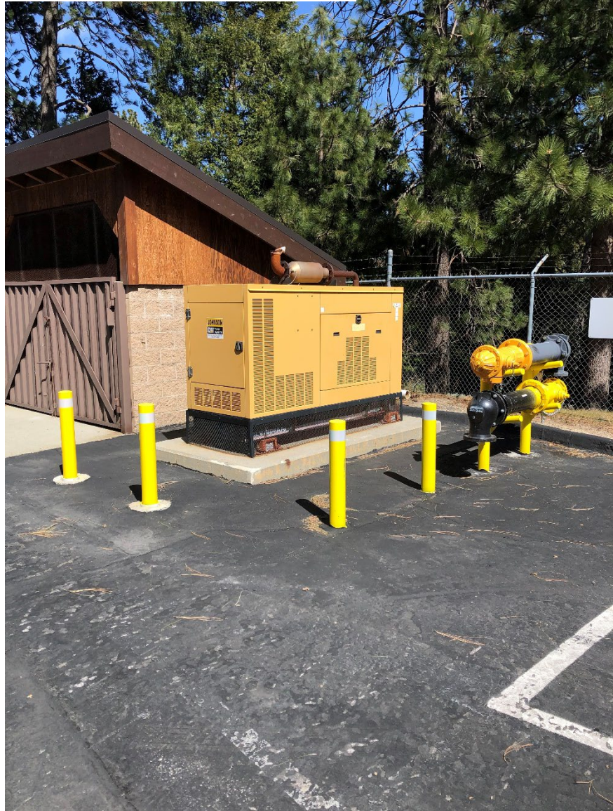
HQ – Emergency Genset Figure 2
