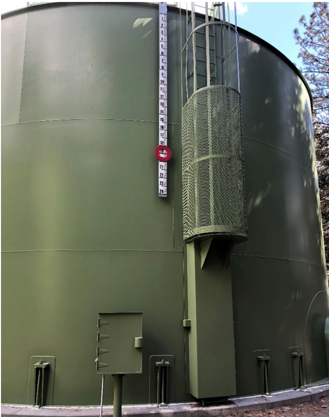
Figure 1 - two tanks, SCADA and data collector
